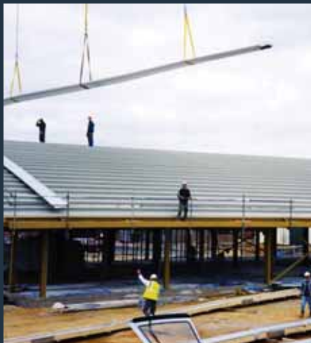
Roofing support system
